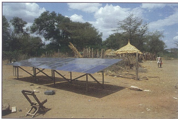
Figure 7.3 This array of solar cells provide electricity for a water pump in a Kenyan village.
